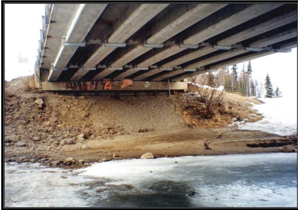
Bridge Abutment at the Chena River Showing Erosion
